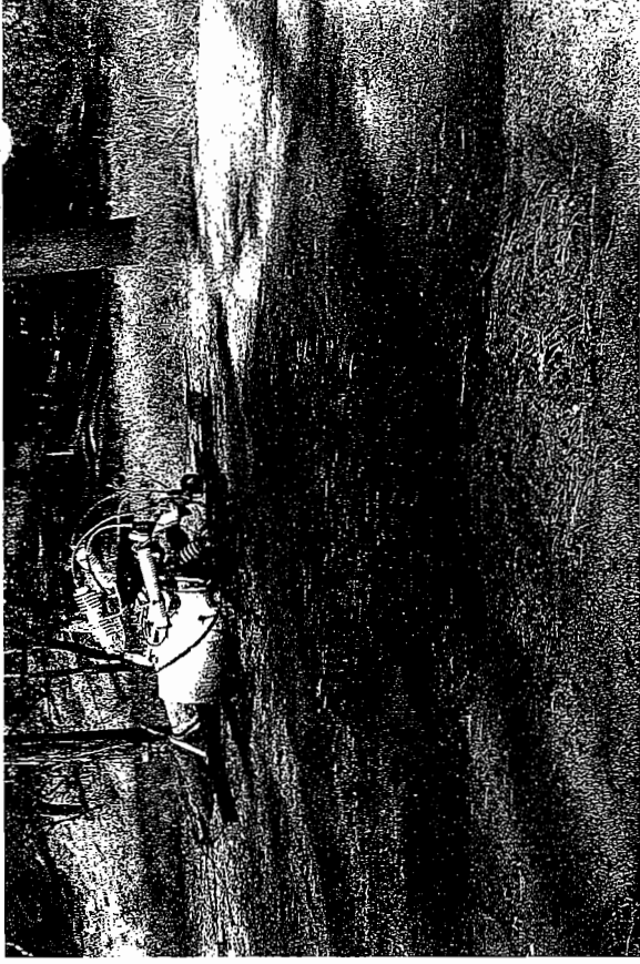
View of fallen power line and transformer and associated staining.
